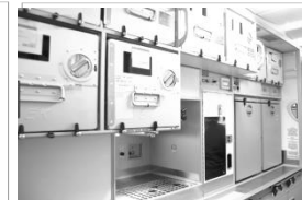
Galley Air Chiller
