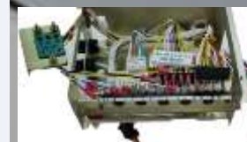
Air Chiller Machine: Electrical Box Harness
