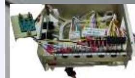
Air Chiller Machine: Electrical Box Harness
