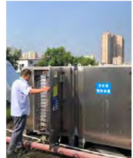
To ensure that waste gases pass through treatment systems before being released into the open air.
