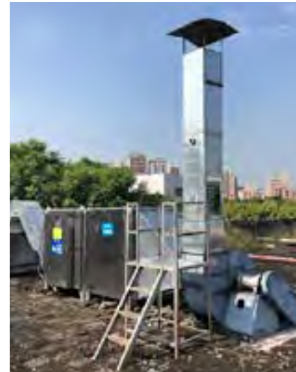
The installation of exhaust ventilation systems, an implementation of 2020 Blue Sky Action Plan.
